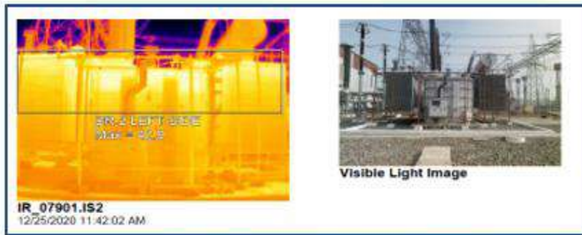
Substation condition monitoring & performance assessment
