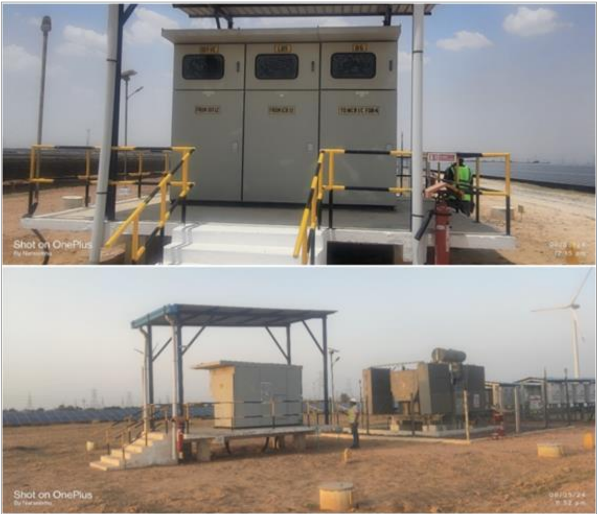
Figure 0-4: Inverter Station and Transformer
