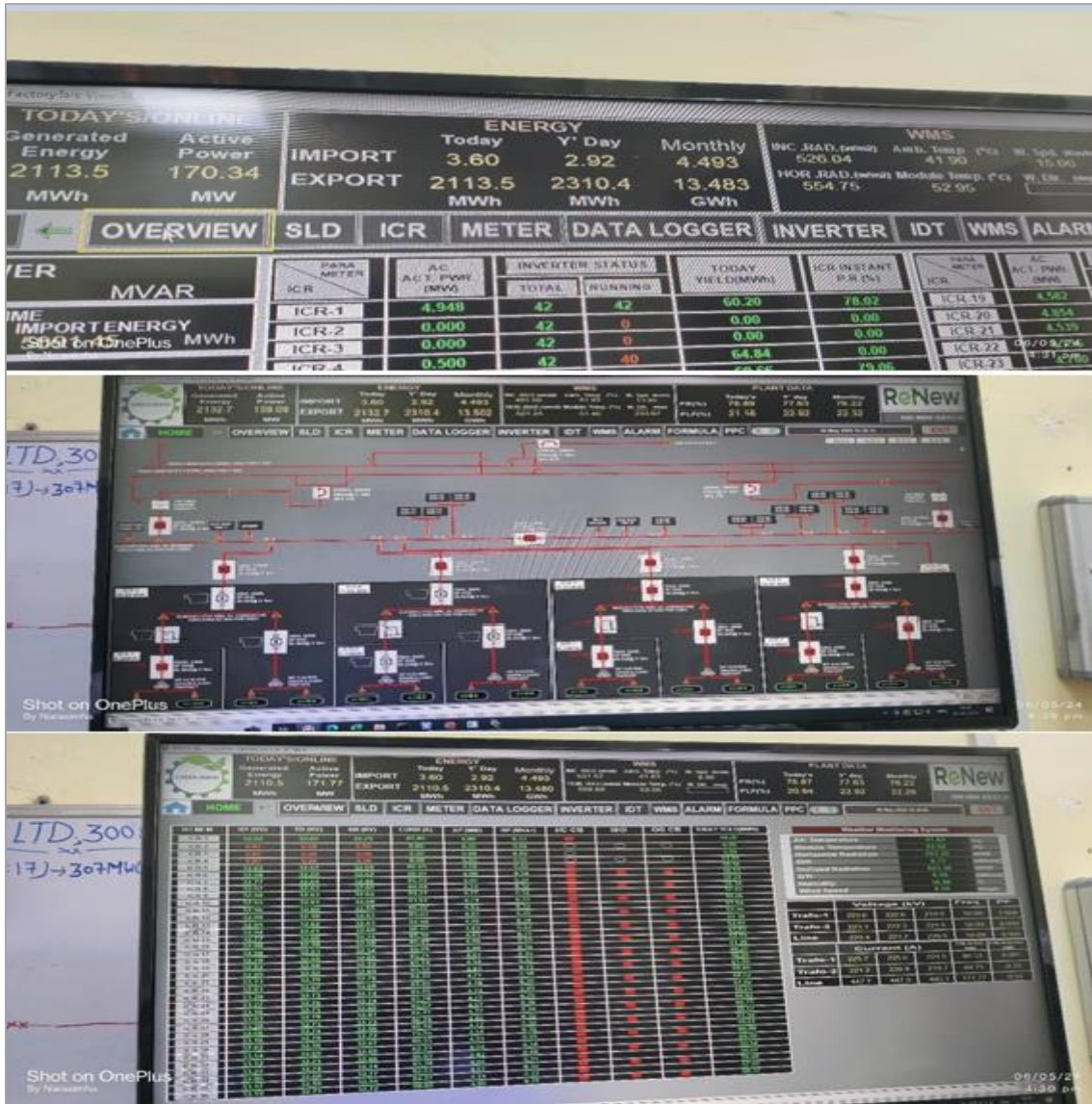
Figure 0-5: SCADA Data System at Project Site
