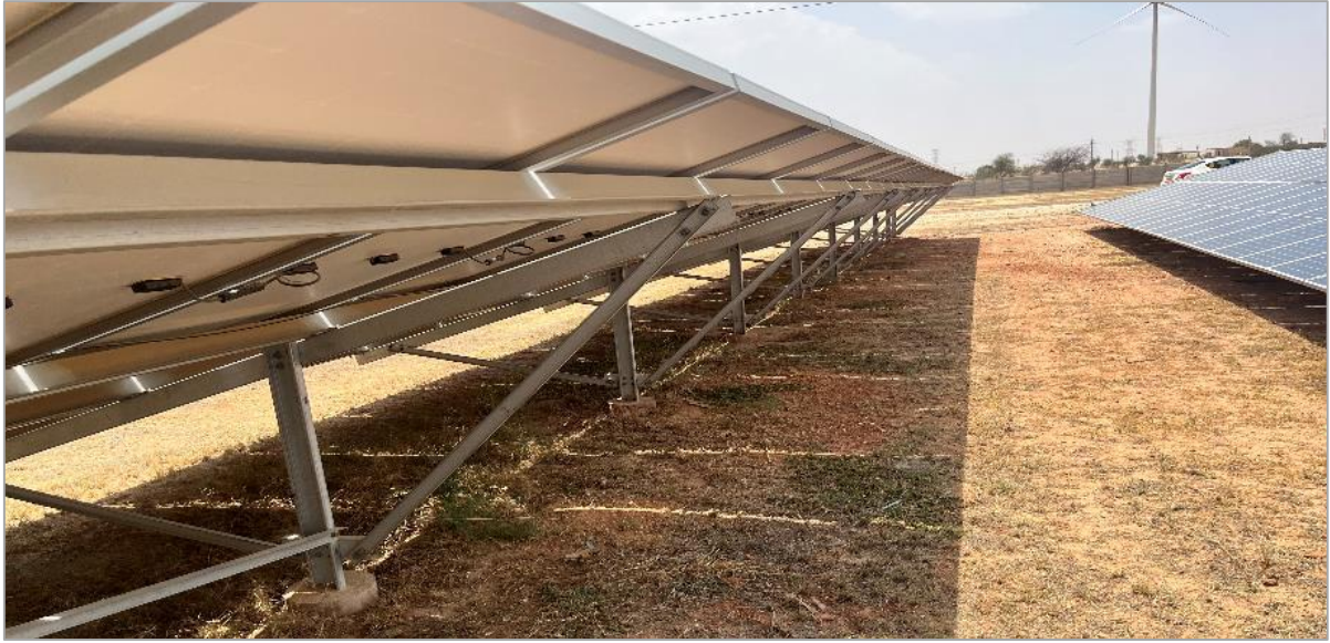
Figure 0-3: Module Mounting Systems Fixed Tilt at Site
